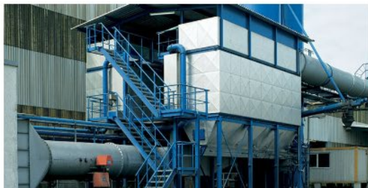
Baghouse Dust Collectors
